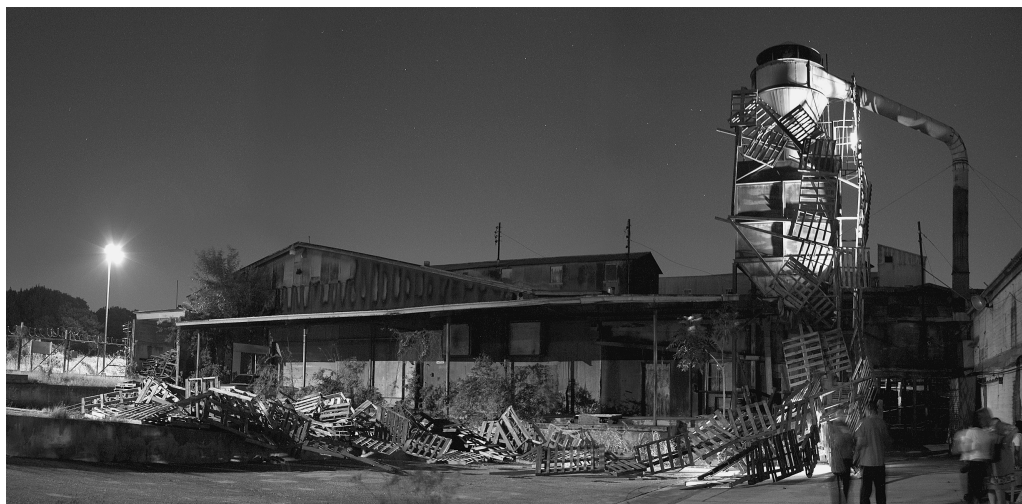
13. Demolition of Site , Planing Building, Friedrich Company Industrial Complex, San Antonio, Texas, 2004. Dwayne Bohuslav and Joanne Brigham, San Antonio College and Houston Community College, respectively. Photo by Ansen Seale.
